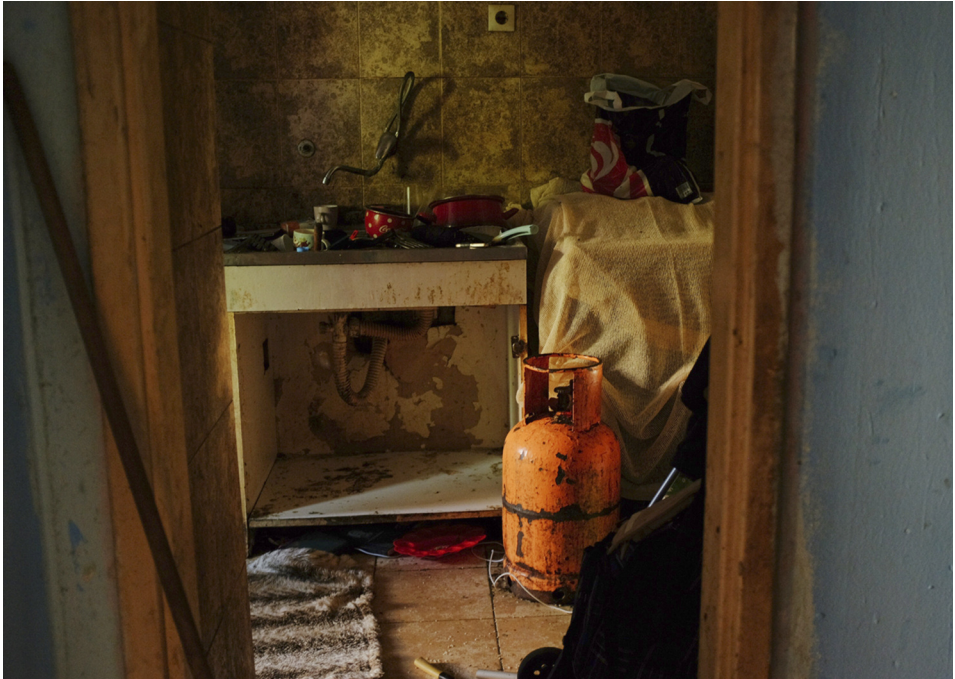
Figure 1: Small kitchen in disrepair with an orange gas cylinder, cluttered sink, and worn surfaces. Author: Sara Nikolić (2024).
