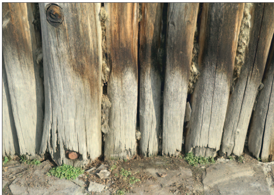
Fig. 3. Modrá. Oak poles of the entry tower embedded in concrete twenty years after construction with legible traces of rain water effects.
