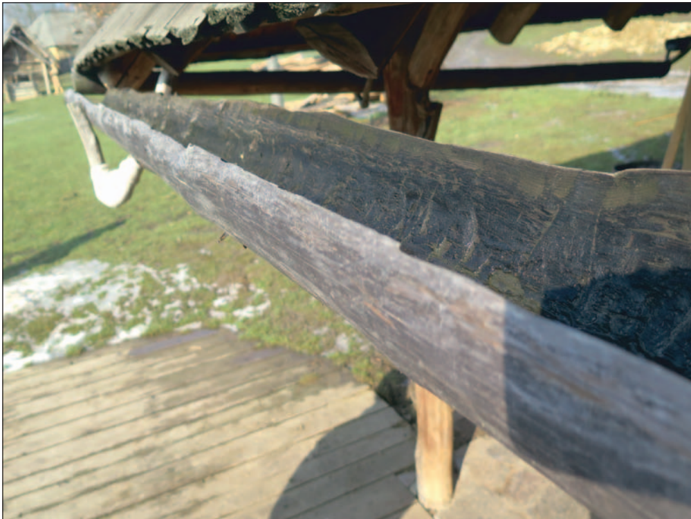
Fig. 9. Modrá. A wooden gutter and its attachment to the lower part of the roof.
