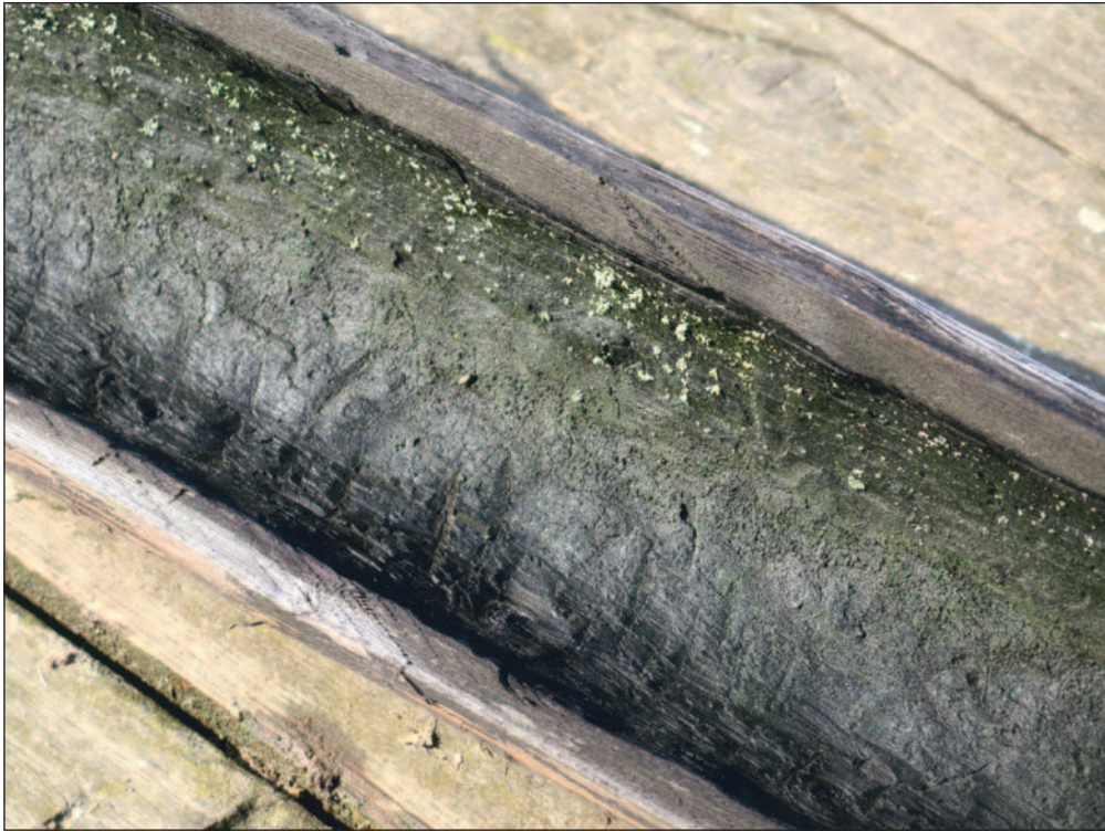
Fig. 8. Modrá. Details of a charred wooden gutter.
